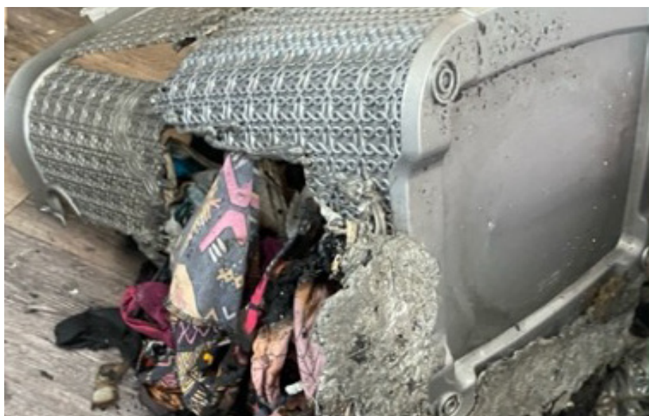
Image Credit Nationwide fire sprinklers, NFRS
