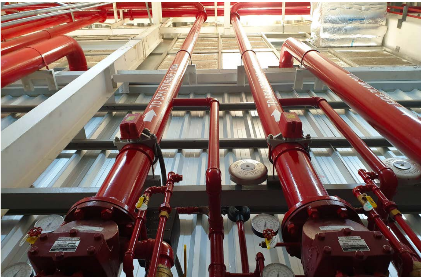
Fire suppression system with an alarm check valve
